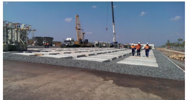
Large above ground storage site
