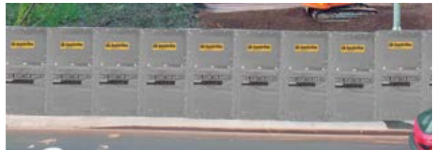
Barriers create a sound-minimizing enclosure between a job site and pedestrian walkway.
