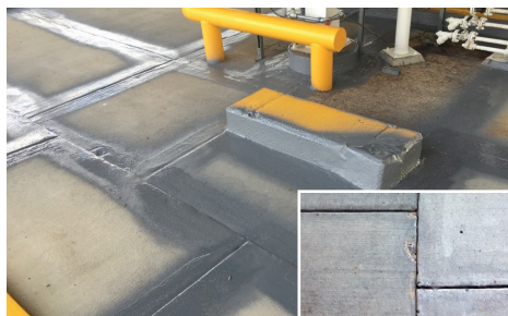
Leak and crack repair
