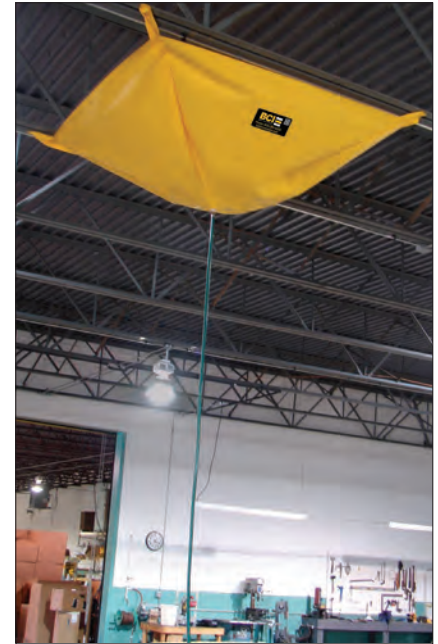
Hose channels rainwater leaks into floor drain or collection container.
