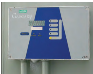
Vapor detection sensors
