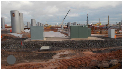
Above Ground Bund
