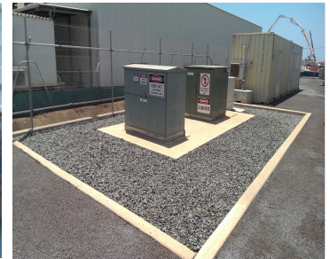
Pad mount for smaller containment.
