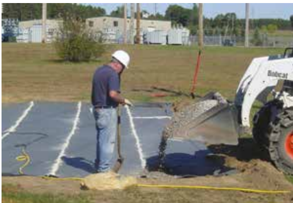
Bentonite clay placed over the seams. Gravel is then placed over the material.
